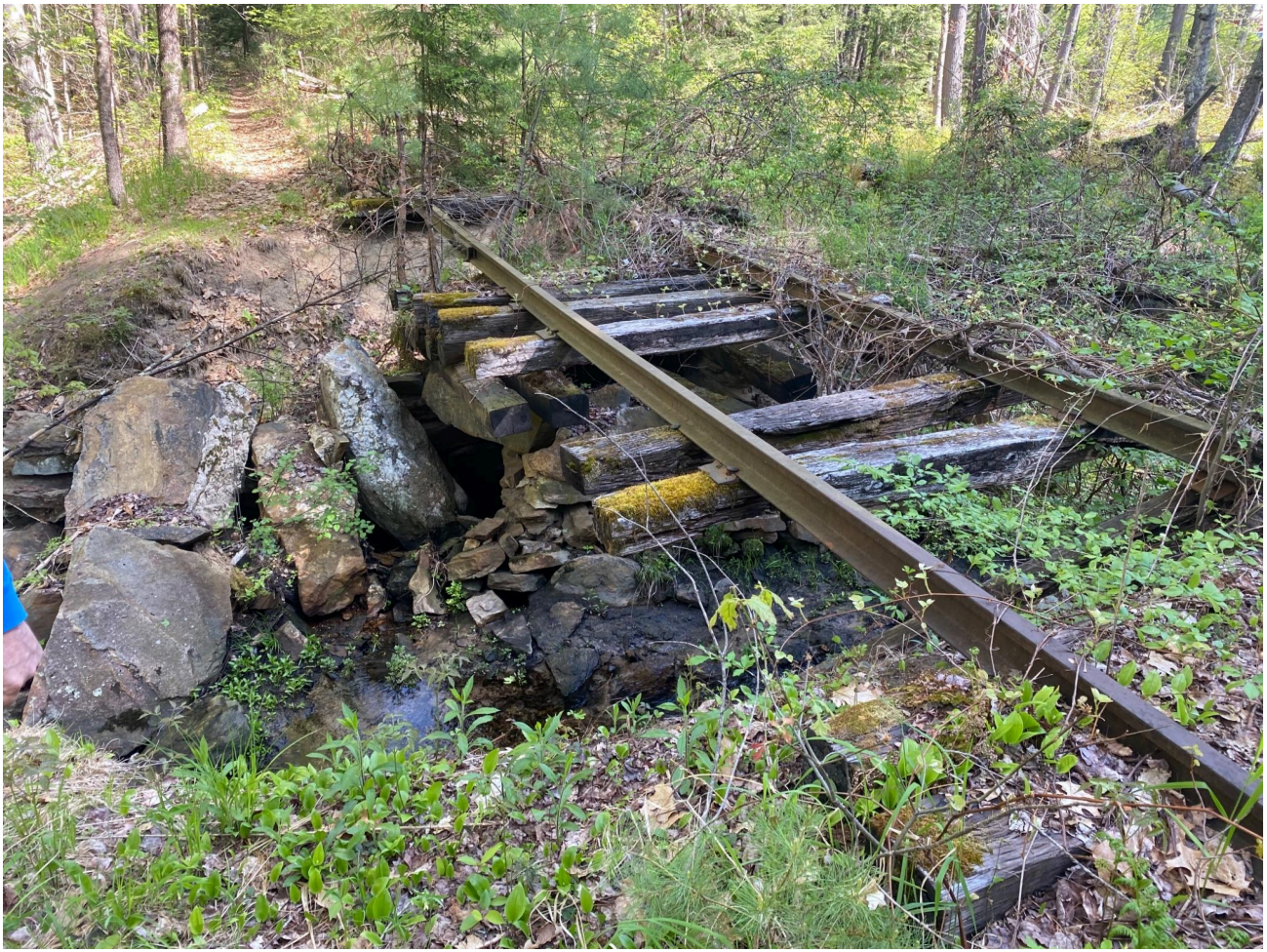
Figure 6: Northern washout in Groton section.
