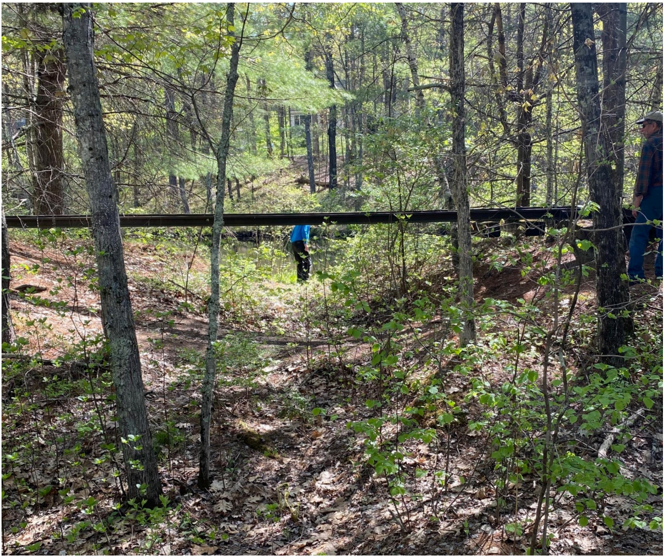
Figure 7: Southern washout in Groton section.
